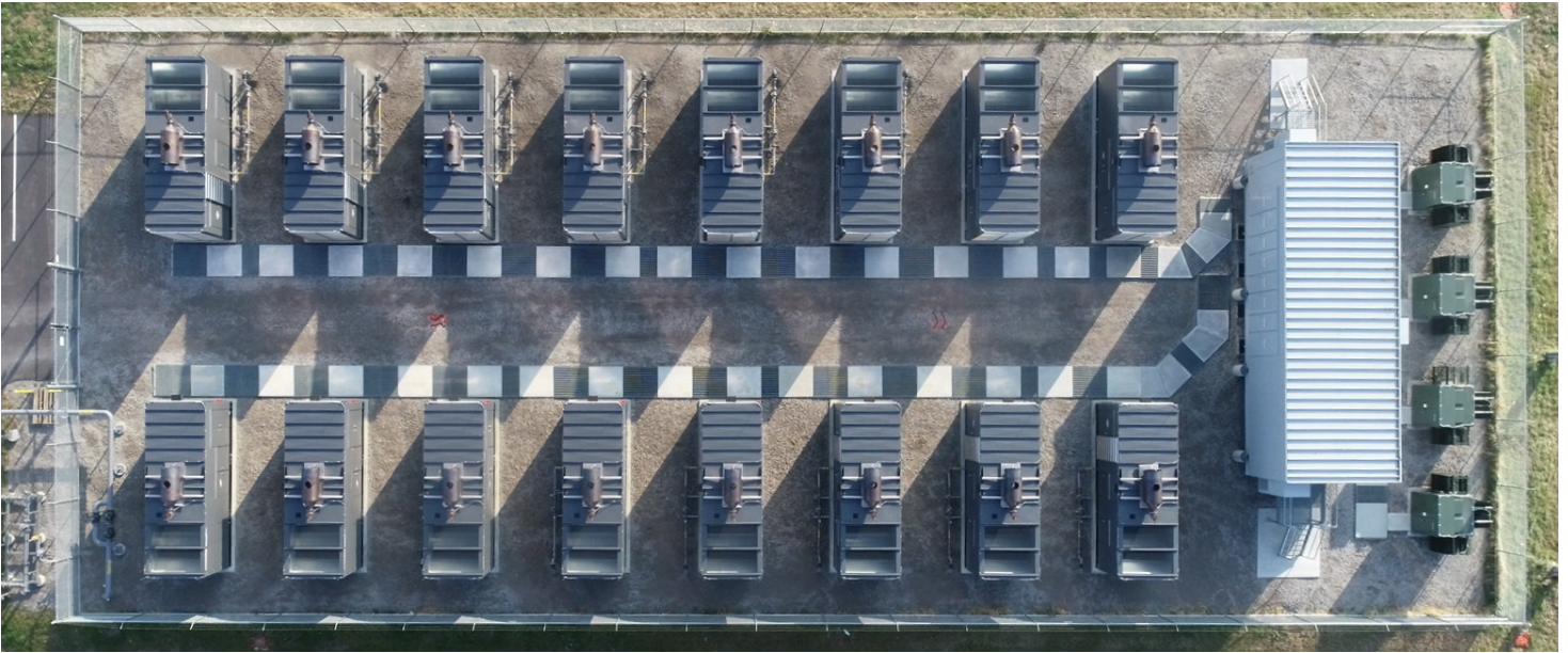
A 10 MWe utility scale microgrid recently commissioned in the midwestern U.S. consisting of 16 x 625kWe natural gas generators.
