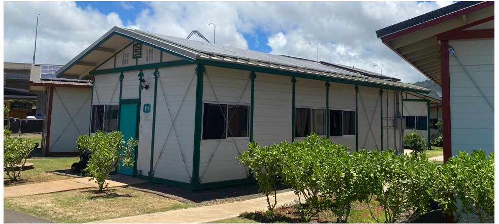
Pictures of the Kahauiki Village microgrid, where a propane generator is integrated with photovoltaic solar panels and battery storage.
